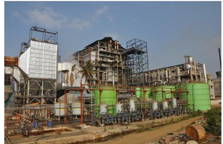
44 MW co- generation plant at Warana, Maharashtra (India)
