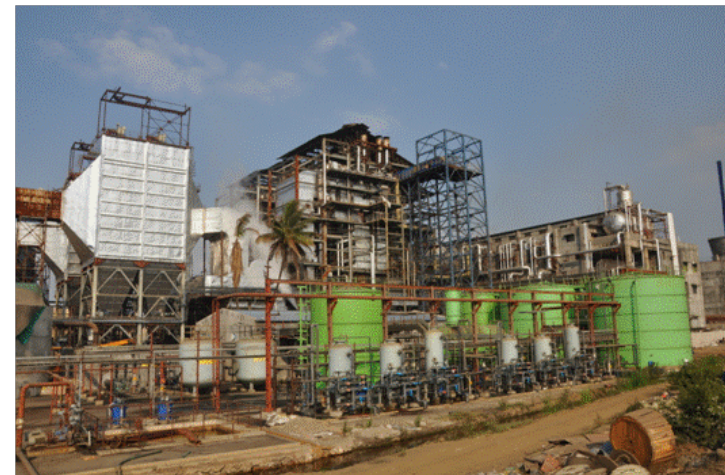
44 MW co- generation plant at Warana, Maharashtra (India)
