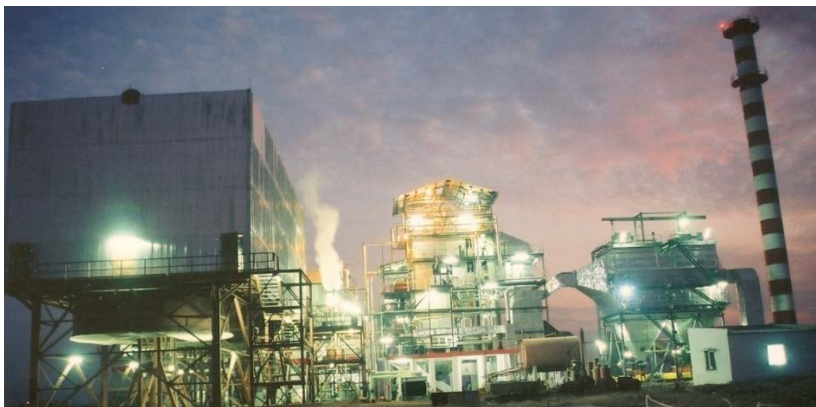
6.6 MW Municipal Waste Power Plant- EPC for Selco International , A.P ( India)
