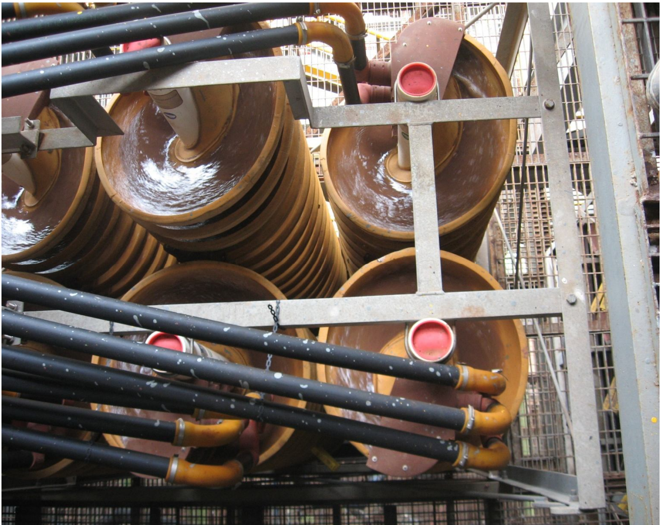
Spirals in Pre-Concentration Plant
